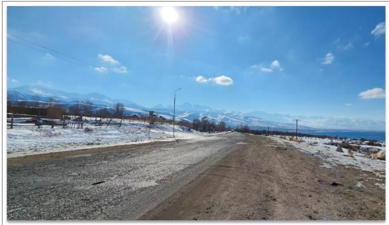
Figure 186– Existing road condition in Jele Tobe
