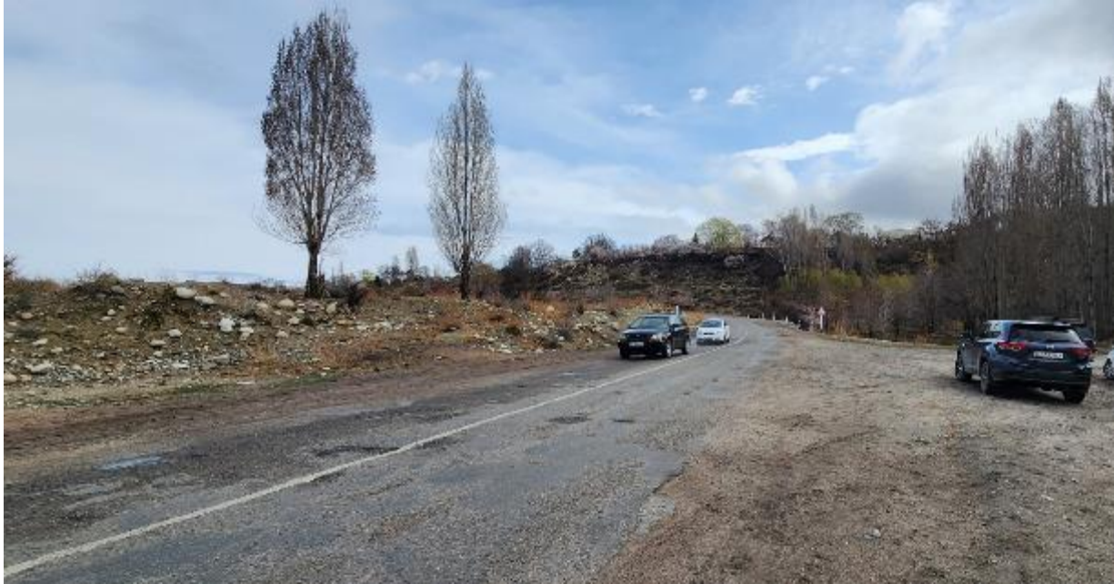
Figure 6: Deteriorated road section near Barskoon
