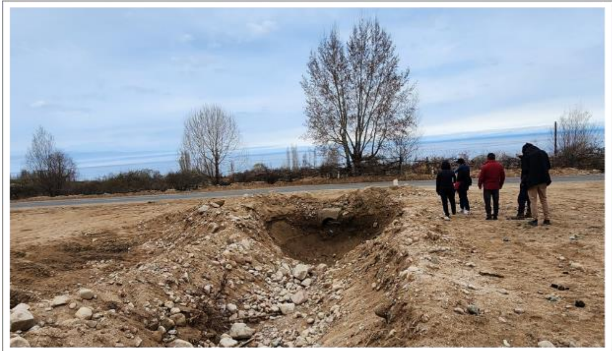
Figure 190: Road section recently affected by flooding near the village of Kichi Zhargylchak (KM 151+70) due to inadequately-sized water pipe/culvert (10 April 2023)
