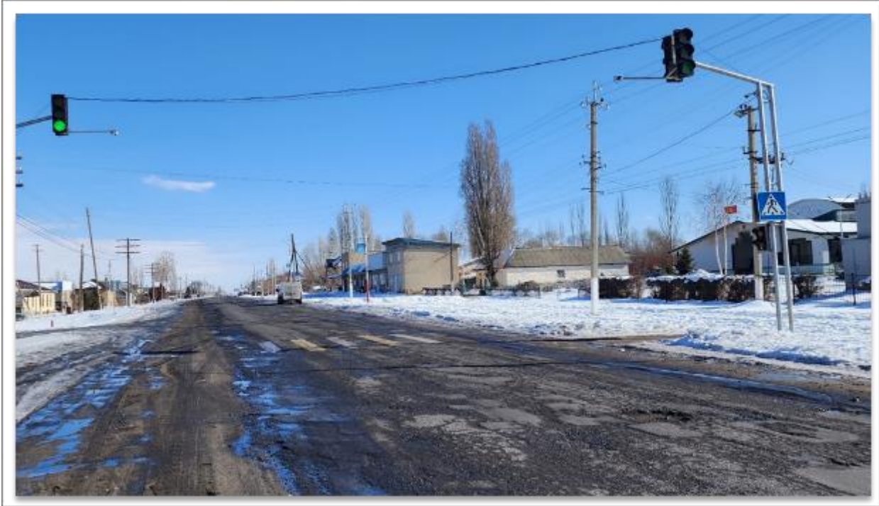
Figure 185– Existing road condition in Darkhan
