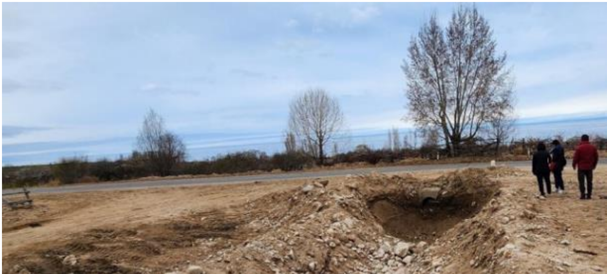
Figure 203``: Road section recently affected by flooding (KM 151+70, 42°12'45.57"N; 77°42'6.94"E) near the village of Kichi Zhargylchak due to inadequately-sized water pipe/culvert (10 April 2023).
