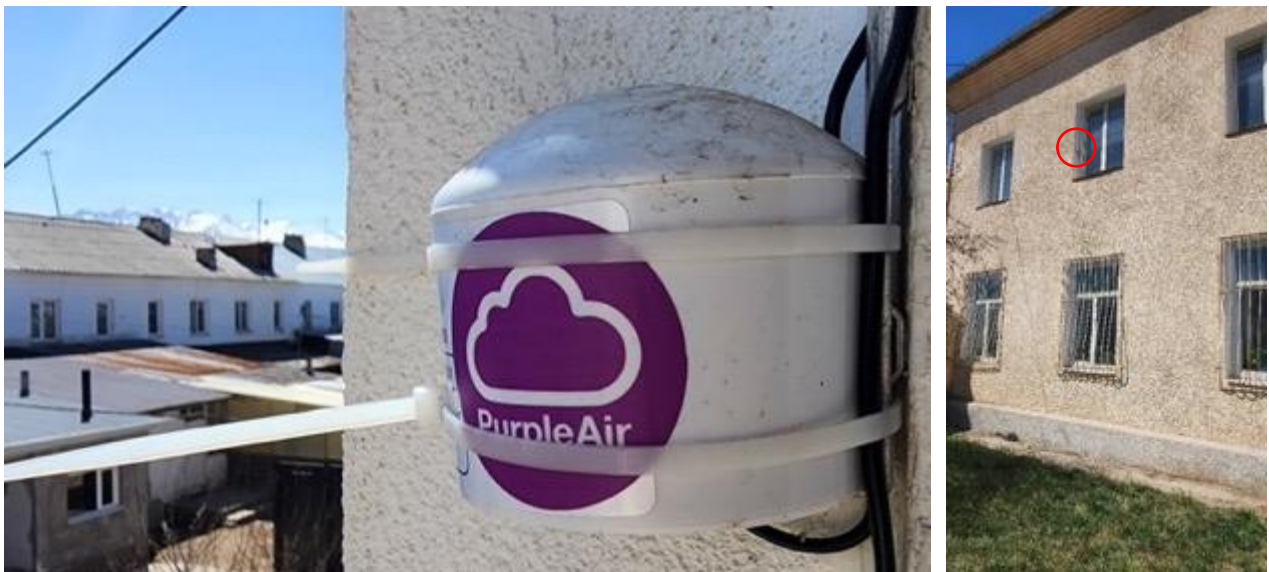
Figure 213: Air quality monitor (sensor) of the Volunteer Organization “Leadership”, installed at the administrative building of the Kyzyl Suu Rayon.
