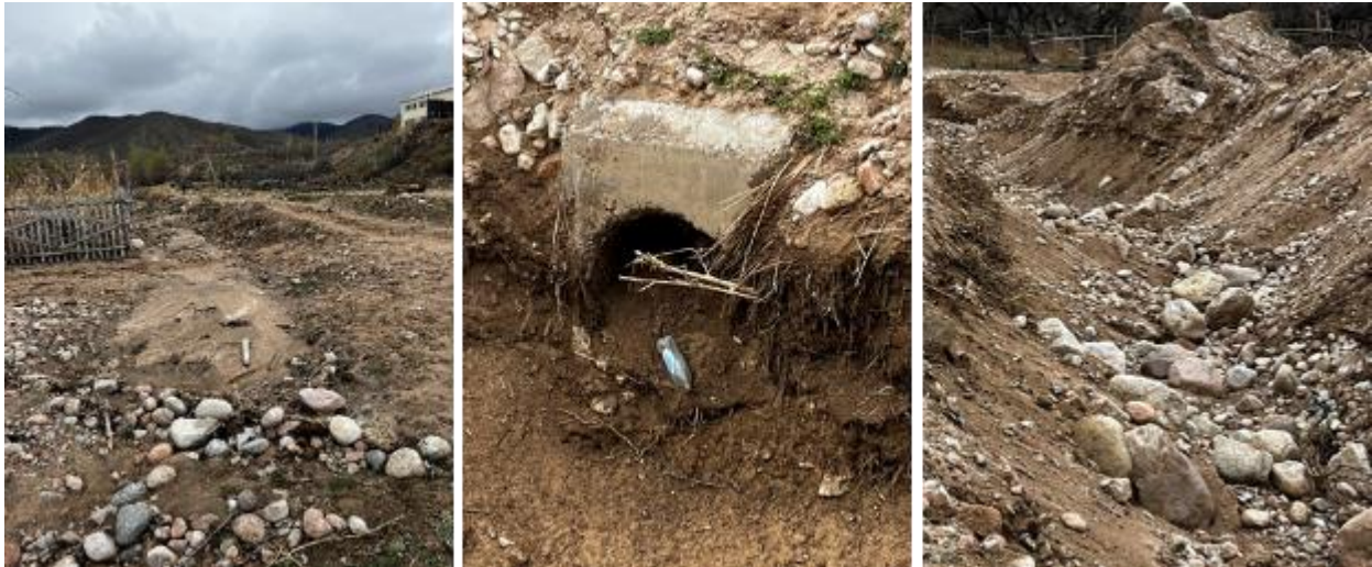
Figure 69: Clogged culvert at KM 155
